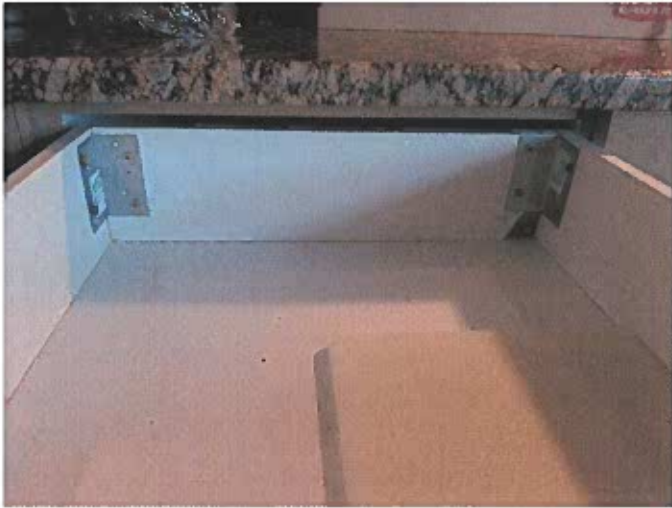
Previous repairs to drawers
